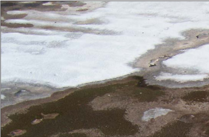
The roofs that were part of the original construction at Ankeney (above), Ferguson and Beaver Creek High School are considered by the OSFC to be in poor condition and need to be replaced.
