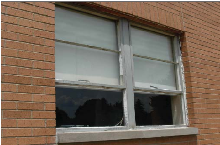
The OSFC noted that the windows at Valley Elementary (above) are in poor condition and need to be replaced.
