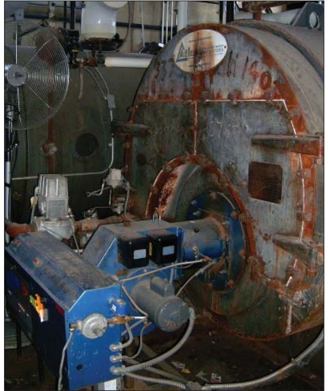
The OSFC noted that the heating boilers at Shaw (above), Parkwood and Valley elementaries are in poor condition and need to be replaced.
